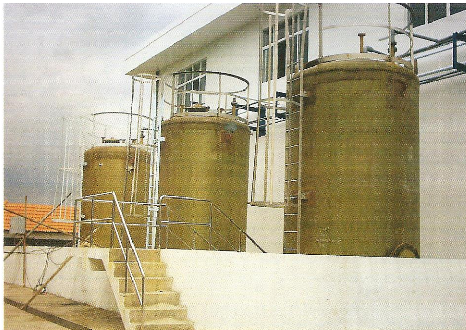
FRP 化學藥劑貯槽 FRP CHEMICAL STORAGE TANK
